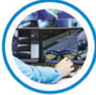
Alarm İzleme Merkezi Alarm Following Centre
